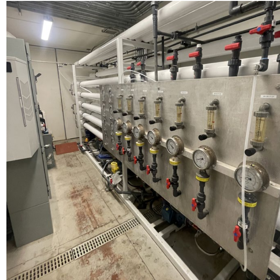
Reverse Osmosis System
